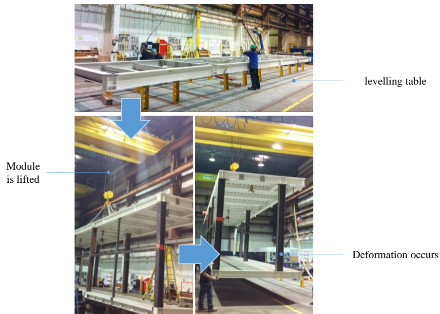
Figure 1-1: Assembly of a parallel system in a fabrication shop. Once module assembly is completed, it is lifted for transportation and shipment. Deformations thereby occur and module assembly on construction site becomes challenging. Photos are taken by the candidate during a site visit in January 2015.
