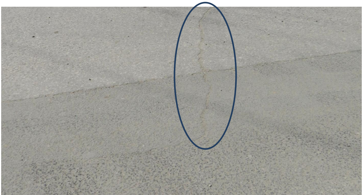
Figure 37 - Photographs of Crack Initiated Outside the Test Section and Ending at the Location of the Perimeter Crack
