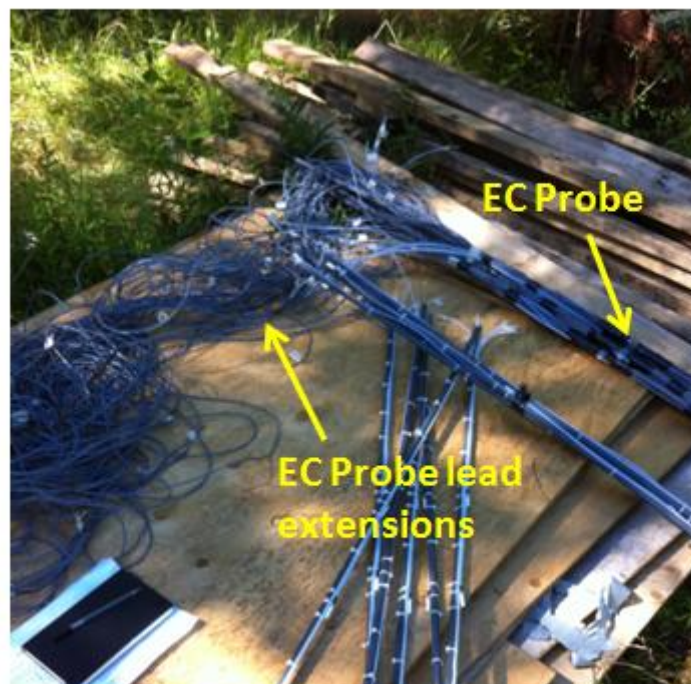
Figure 2.10: Field resistivity probes attached on the EC multilevel. Resistivity probe leads extend to the ground and connect to the data logger.
