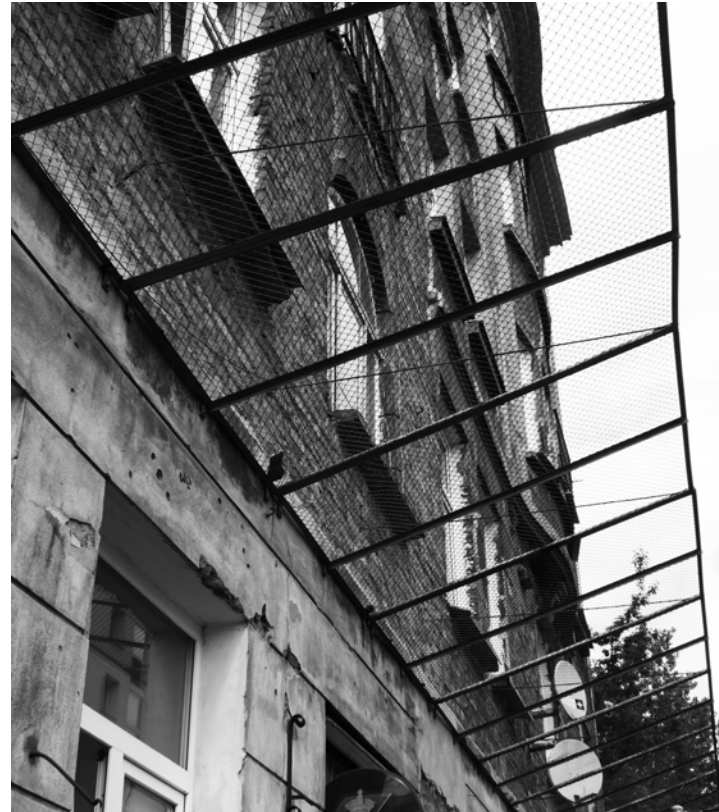
6.6. Provisional solutions to crumbling brick.
