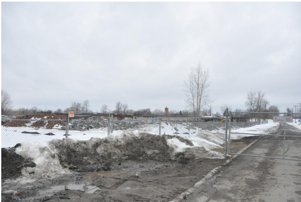
Figure E-4: Site photo of CLC Rockcliffe Lands viewing the former school building that is currently undergoing demolition. The roadway
