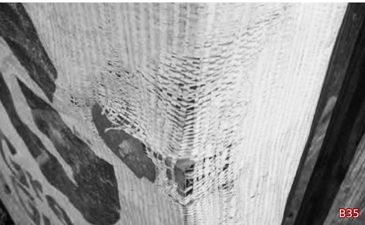
Image B35 (above) Photograph from Office of Inspector General's Audit of USAID's Efforts to provide Shelter in Haiti. USAID was required to build temporary shelters that lasted 3 years, this tarp exterior failed after 3 months. 18
