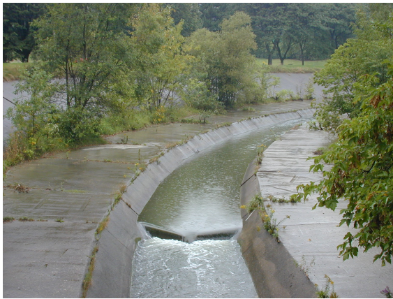
(a) Concrete channel with control
