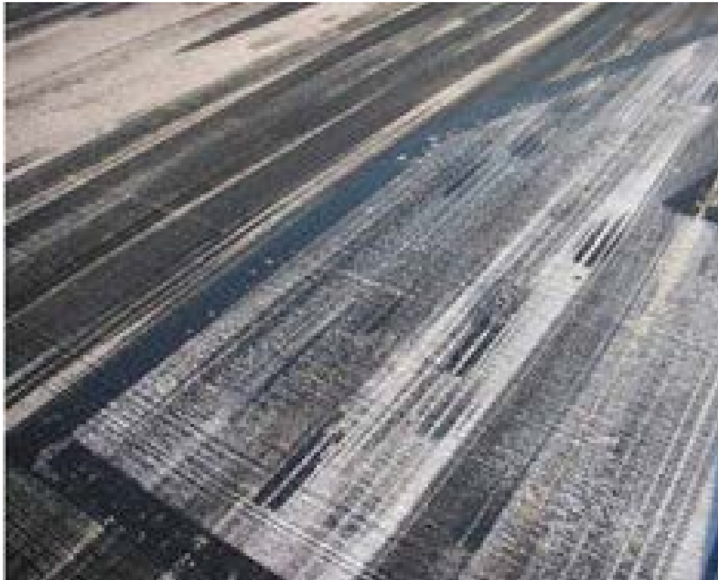
Figure 4.1 - Rubber Buildup on a Runway [Bangkok, 2008]
