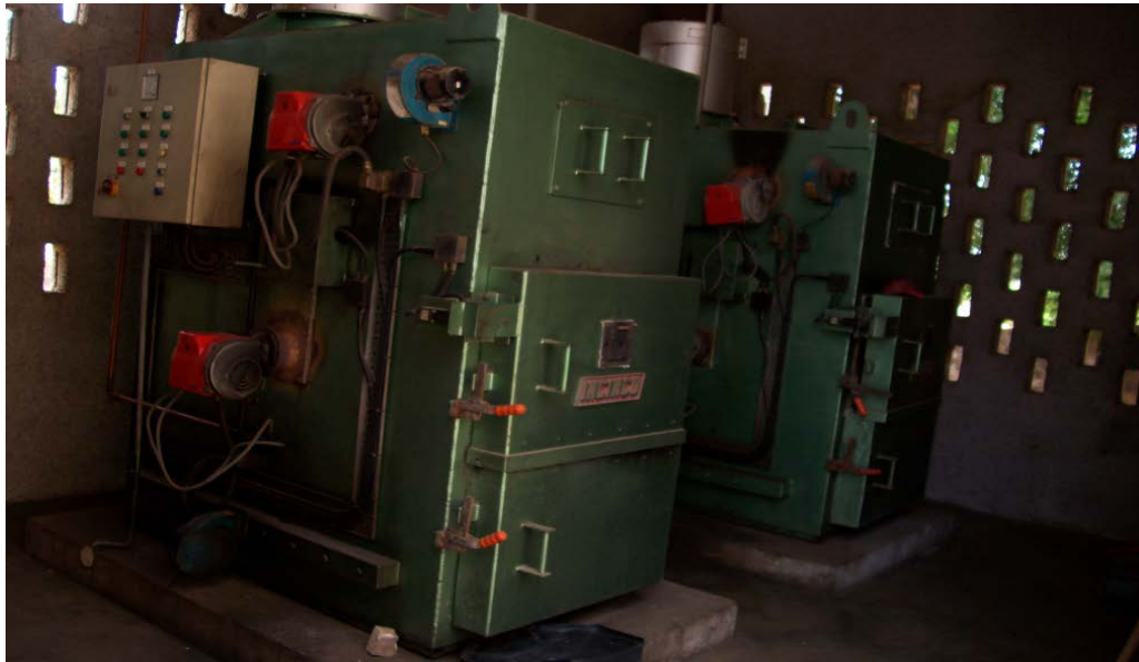
Figure 7.10: Onsite incineration technology for treating anatomical residue in a healthcare facility in the AMA. Photo by Squire, 2010
