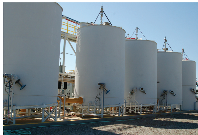
Fig 2.39 Onsite Power System's demonstration Anaerobic Phased Solids digester system located at University of California at Davis.
