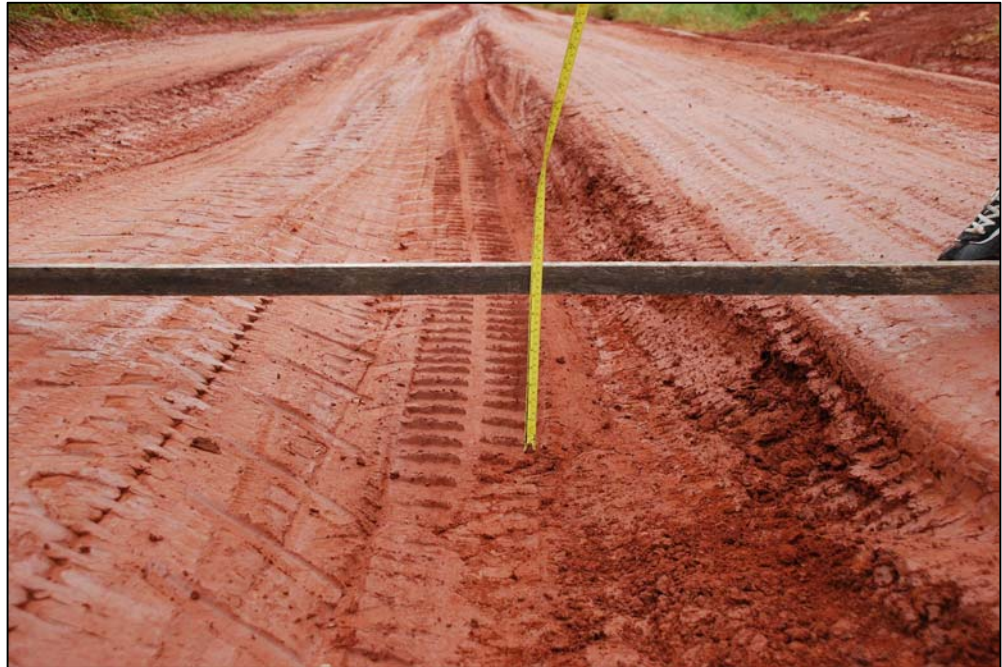
Figure E.4.2 Severe Rutting in Road 2.1
