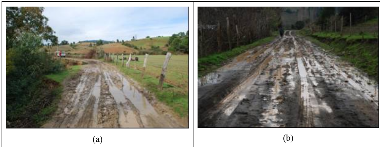
Figure E.1.3 Drainage Problems in Roads (a) N498 and (b) Local Road V_LLA
