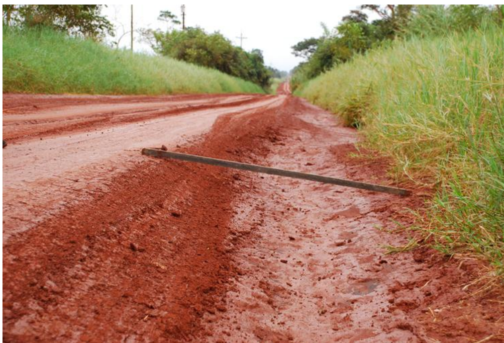
Figure E.4.4 Erosion in Road 11
