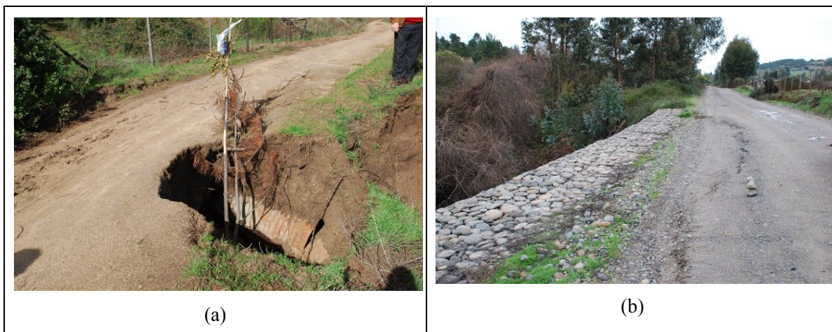
Figure E.1.4 Erosions Caused by Unstable River Banks and Drainage in Roads (a) N474 and (b) N620
