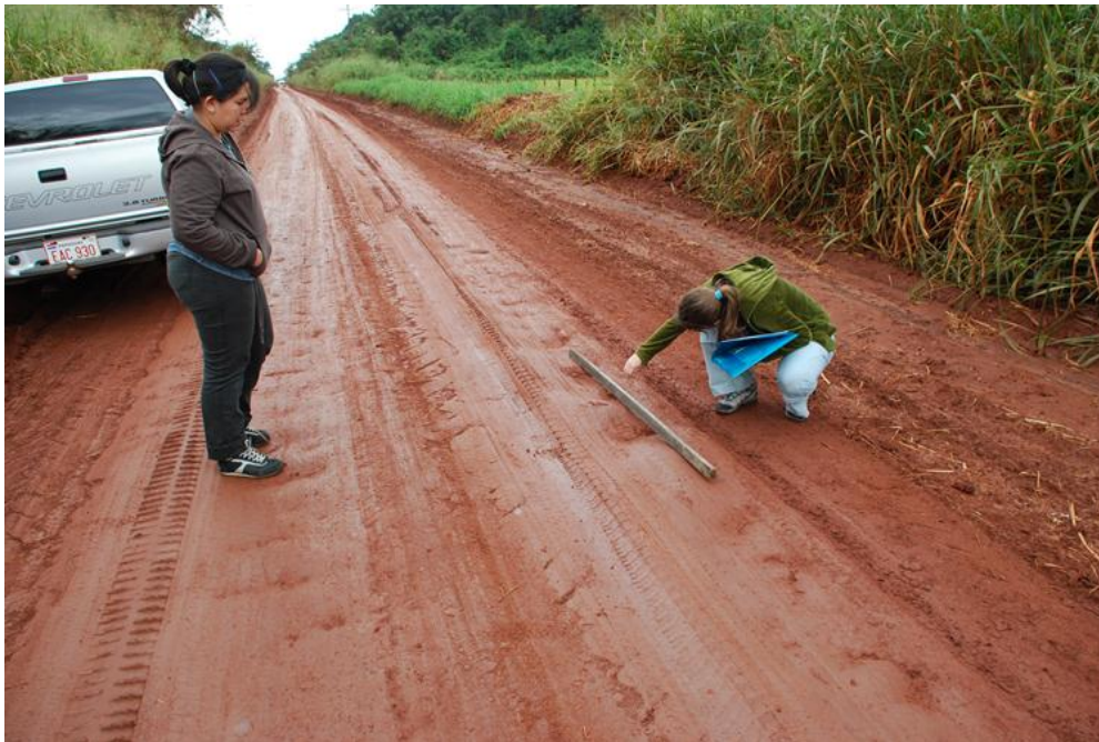
Figure E.4.3 Fixed corrugations in Road 9
