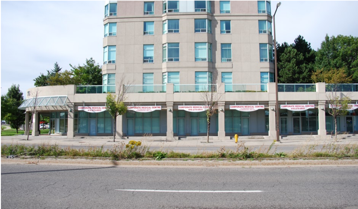
Fig. 3.5 The modern condo podium contains commercial units, but fails to attract a mix of tenants and generate pedestrian activity
