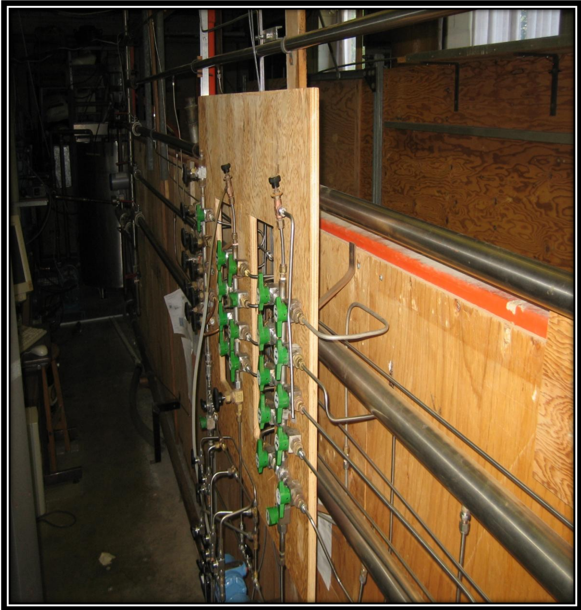
Figure 4-2: Pipeline flow loop
