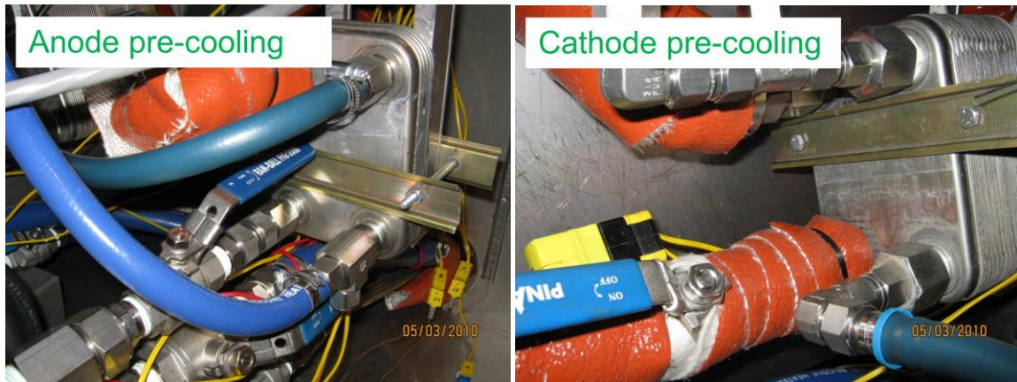
Figure 0-4: Gas reactant pre-coolers
