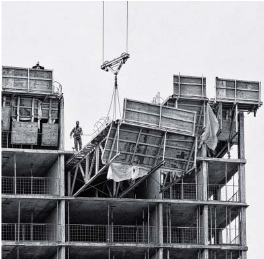
» fly-forming in progress. The form is being craned from one floor to the next above. [above]
