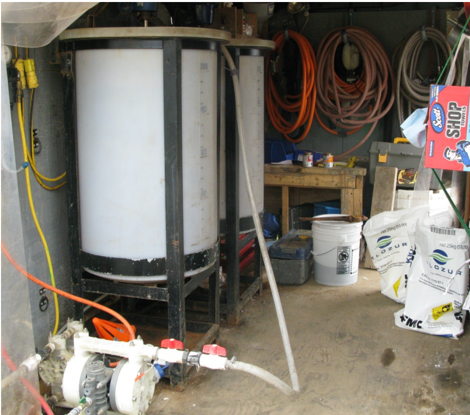
Figure 38 - Mixing tanks for oxidant solution
