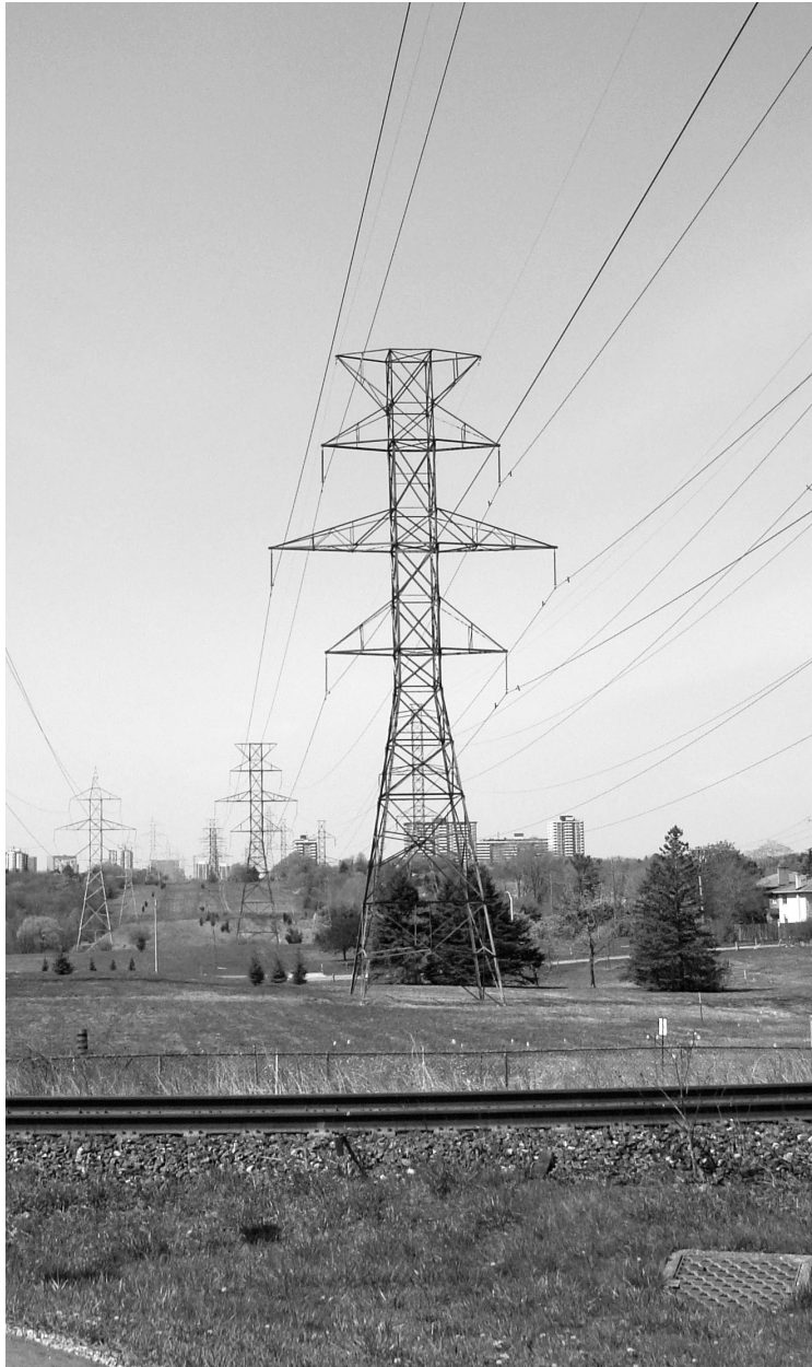
Fig.3.2 Looking west along Toronto's Finch Hydro Corridor from GO Transit's Old Cummer Station.
