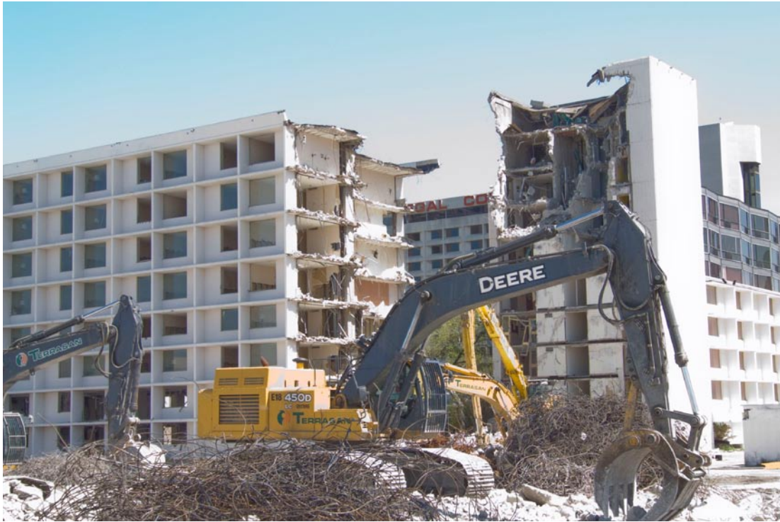
fig. 2.02: Demolition of Constellation Hotel, Etobicoke, ON; showing on-site material recovery operations, separation of reinforcing steel from aggregate. Photo by author, 2008.
