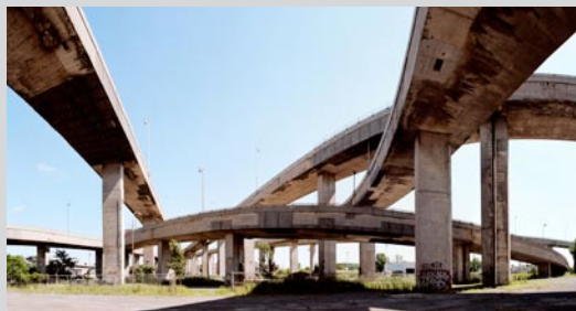
fig.5.01: Deteriorating infrastructure at Turcot Interchange. Photo by Author, 2007.
