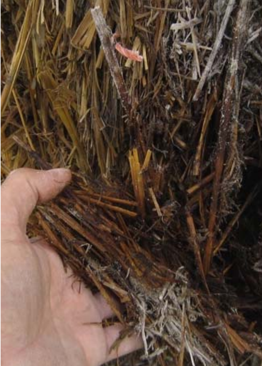
Figure 82. Photograph showing the highly decomposed straw on the right side of the cement-lime plastered wall.
