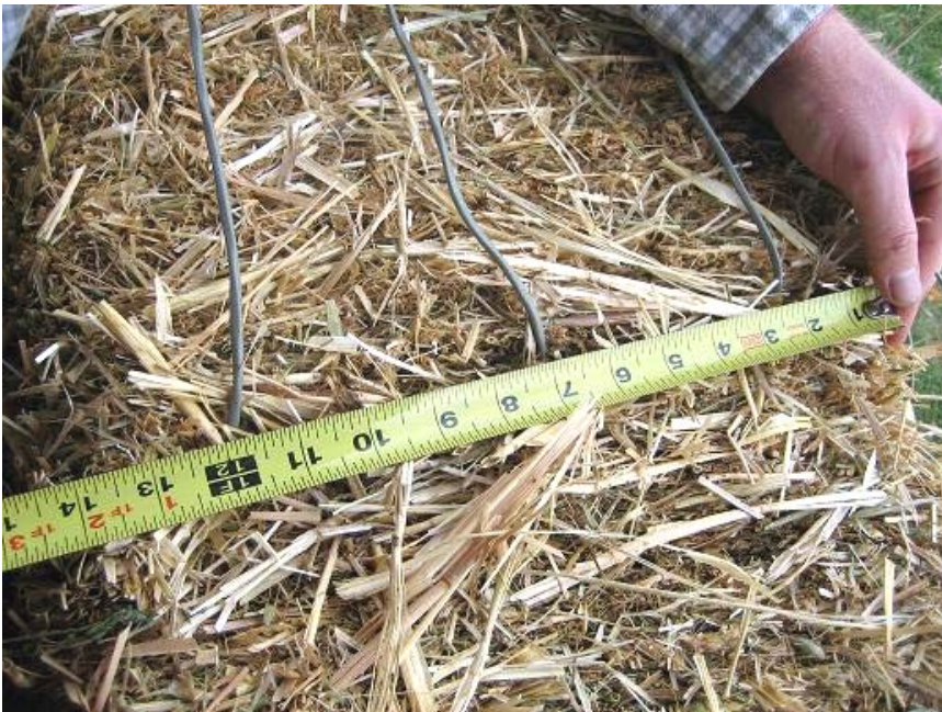
Figure 86. Installation of mid-height sensors in the earth plaster wall showing bale thickness greater than 14".
