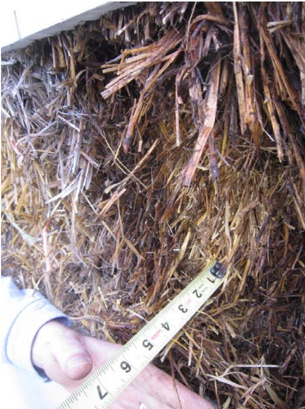
Figure 84. Depth in inches of the highly decomposed straw in the cement-lime plaster wall.
