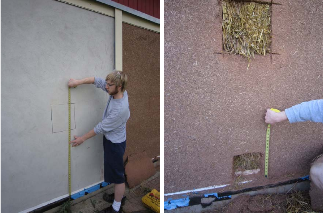
Figure 77. Location of cement-lime plaster removed (left) and clay plaster removed (right) on June 15, 2010 for mould inspection.
