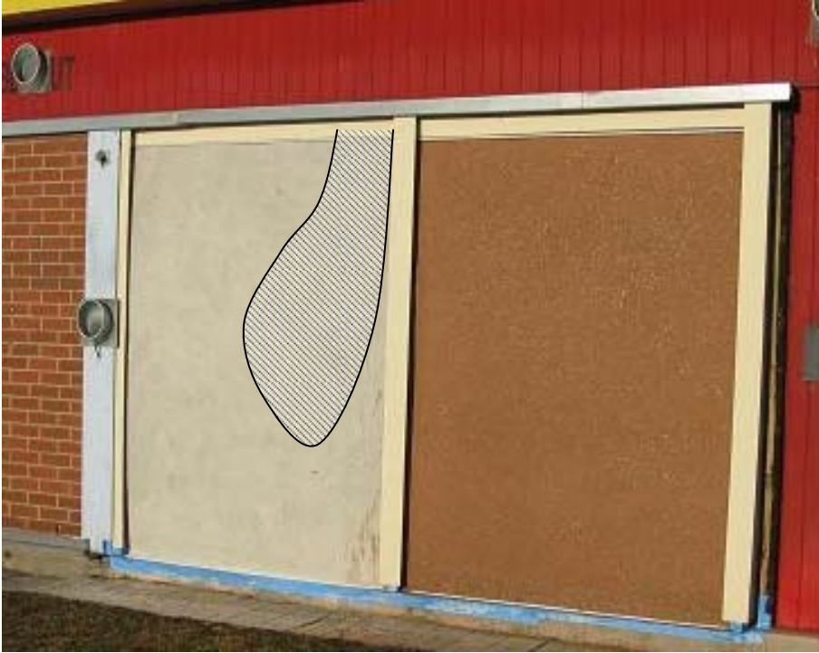
Figure 83. Extent of the highly decomposed straw in the cement-lime plastered wall.
