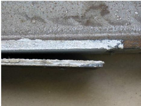
(a) Peeling off action at the end of CFRP strip)
