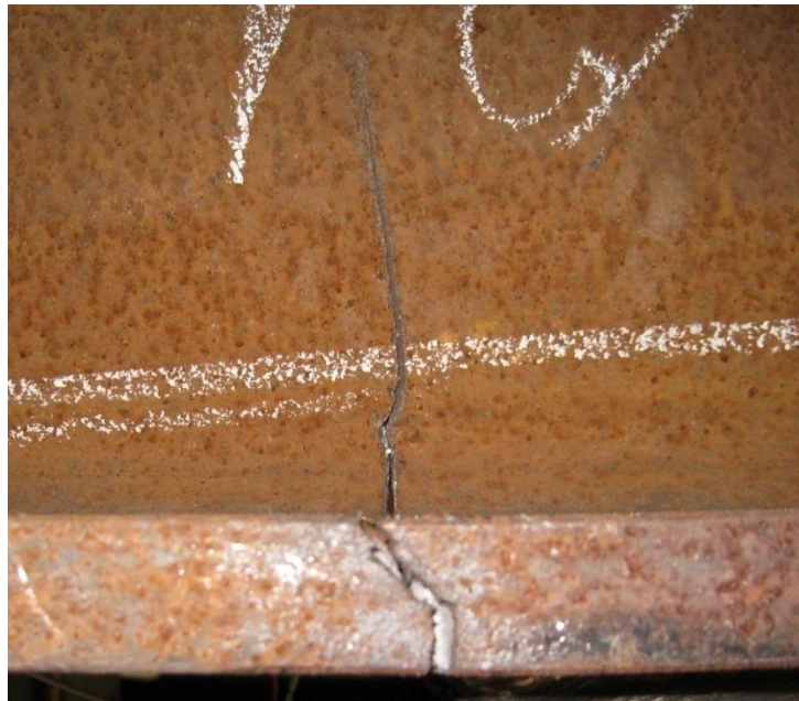
Figure 4.23. Crack from the flange to the web of control specimen
