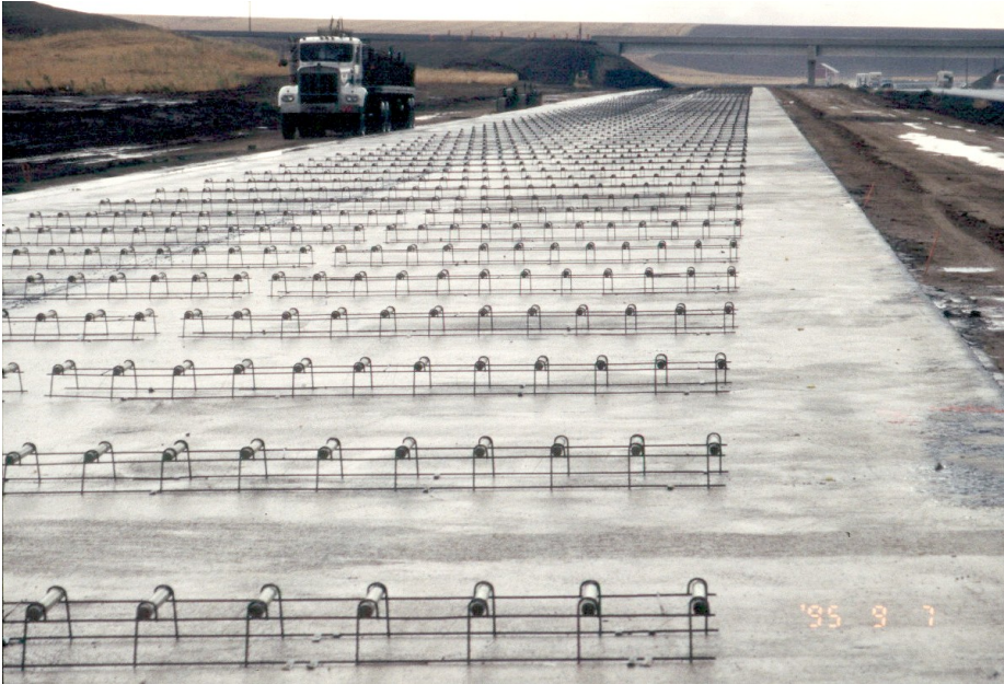
Figure 2.2: Dowel baskets placed on a lean concrete base in advance of PCC placement [10]
