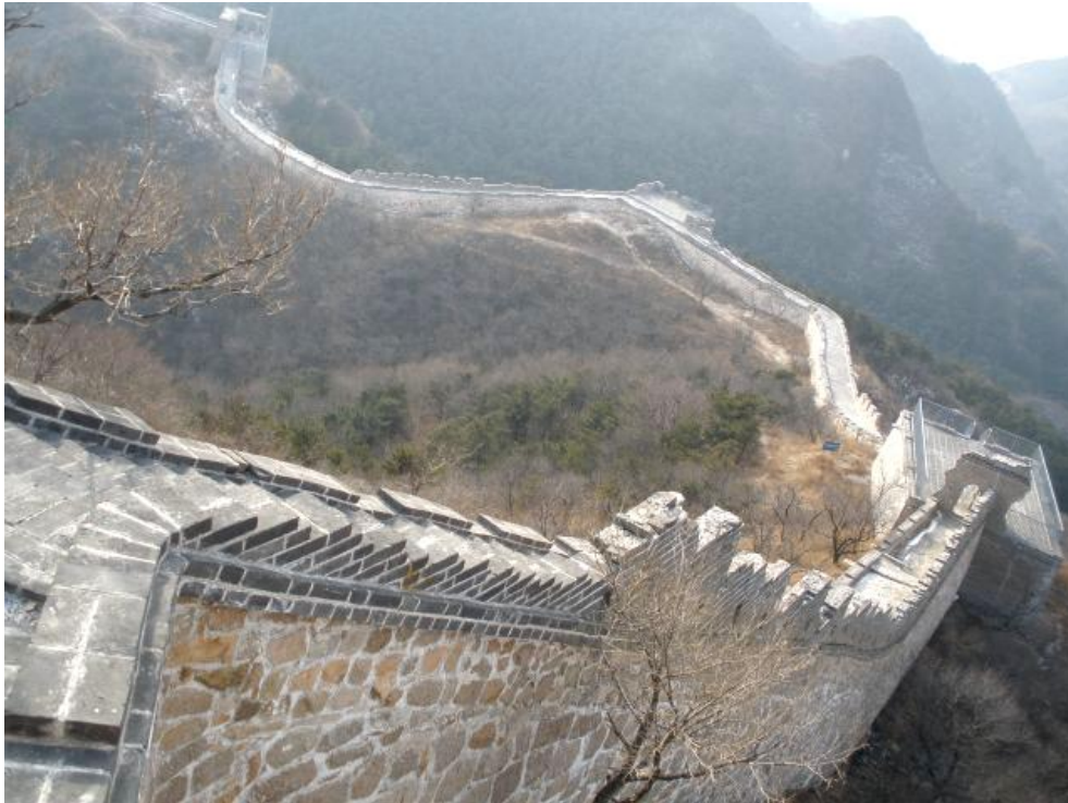
Figure 5.7: Un-renovated Great Wall at the south end of Badaling
