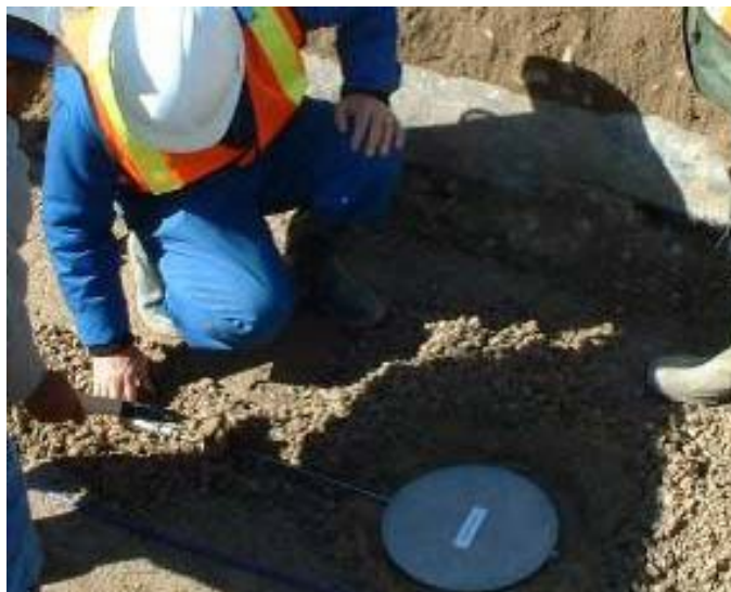
Figure 3-4: Placement of Total Pressure Cell (Adedapo 2007)
