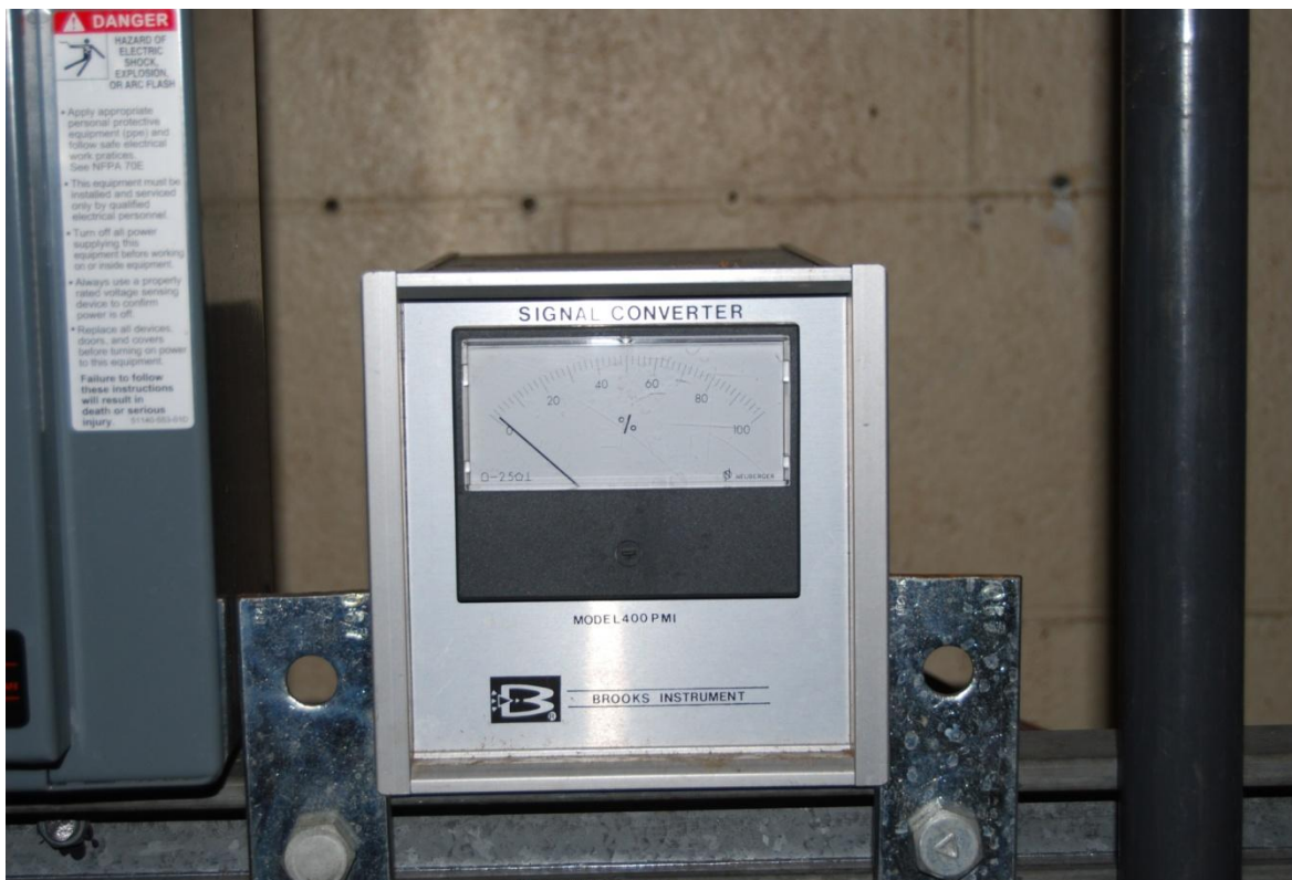
Figure 4.6 View of the liquid flowmeter and its signal converter
