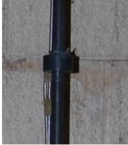
Figure 4.16 View of pressure tap on 1/2" pipe
