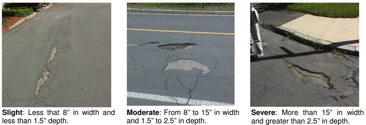
Figure 2.7: Severity Level of Pavement Cracks
