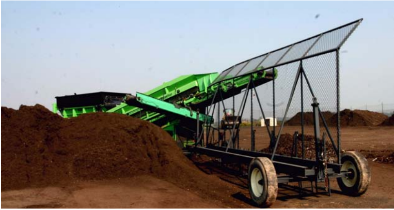
fig. 1.32 Mobile material sorting, processing, and screening operation — Demand for soil remediation is encouraging design innovation
