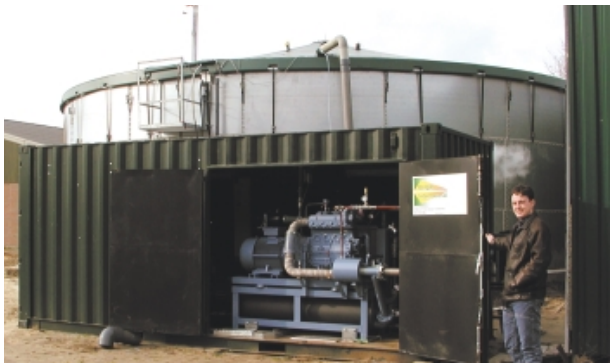
fig. a3.8 Biogas plant for manure digestion Praktijkcentrum Sterksel, The Netherlands
