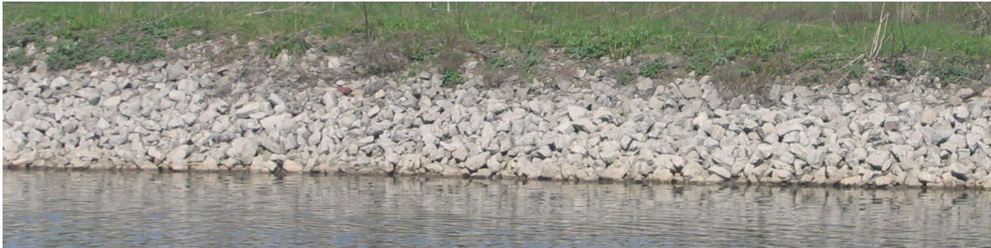
fig. 3.27 The banks of the mouth of Red Hill Creek and Windermere Basin use extensive rock supports — Learning from the Fort Devens Reclamation project there is opportunity to redevelop these banks with extensive reconstructed bio-engineered banks. Doing so will create habitat for plants and animals while improving water quality.
