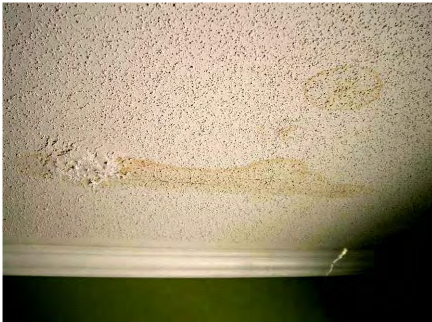
Figure 5.5 – Moisture damage on bedroom ceiling
