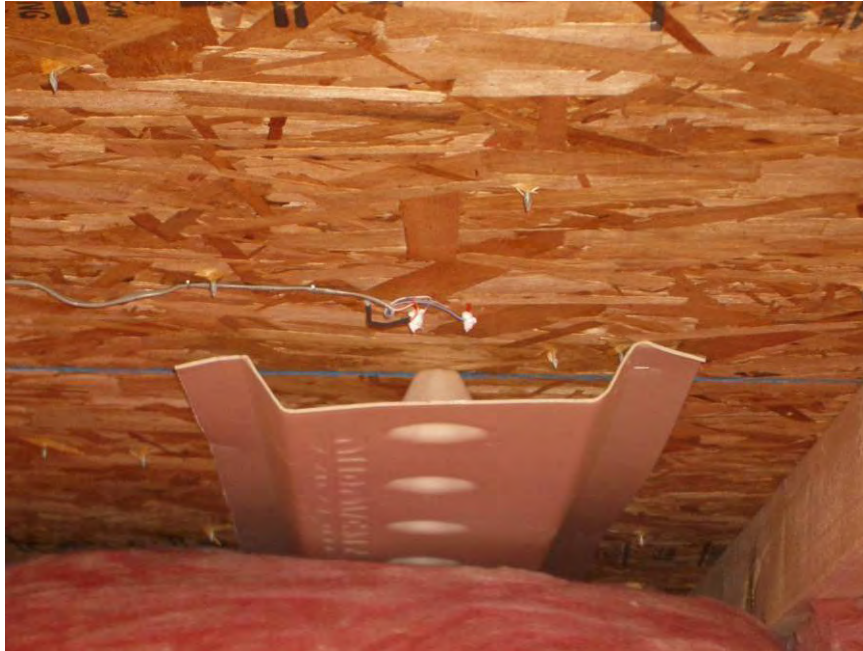
Figure 5.39 – Moisture content pins and sheathing temperature at ventilation chute
