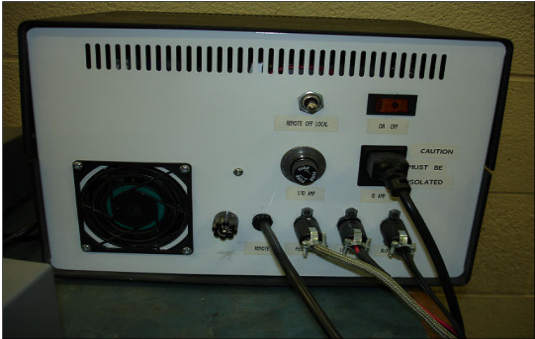
Power Supply Cabinet for Lamp Feedback Mechanism
