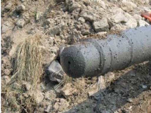
Figure 6-13: Condition of Carrier Casing After 2 nd Pullout.
