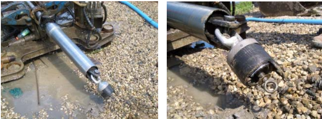
Figure 6-25: The Broken 100-mm Pipe after the Second Pullback Attempt for West Well
