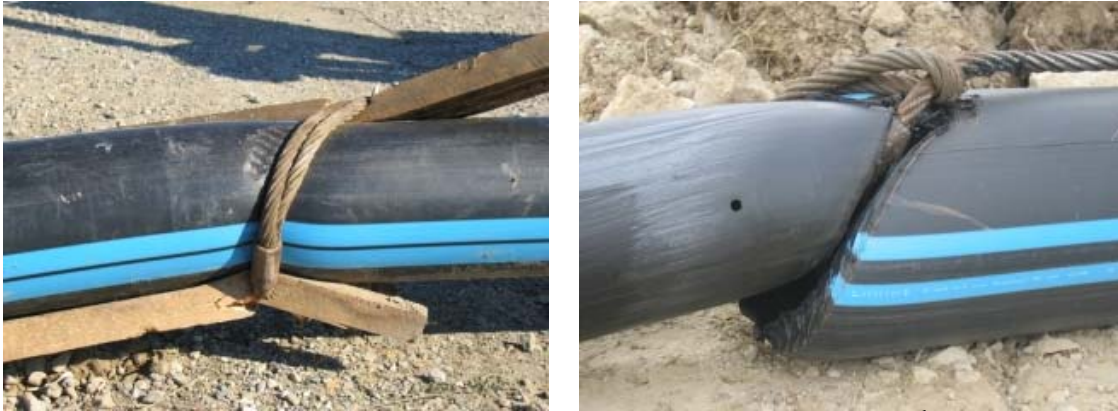
Figure 6-16: Damages on the 200-mm and 150-mm HDPE pipe after 3 rd Pullback Attempt.
