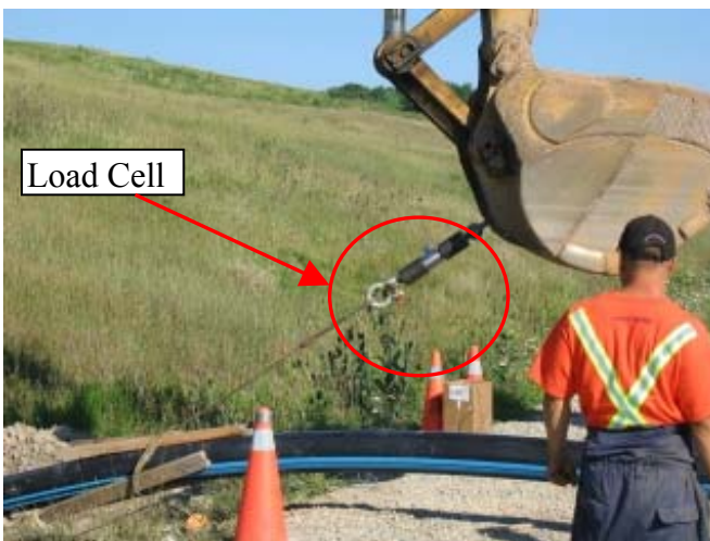
Figure 6-12: Load Cell Connected to the Excavator during 2 nd Pullout of Carrier Casing.
