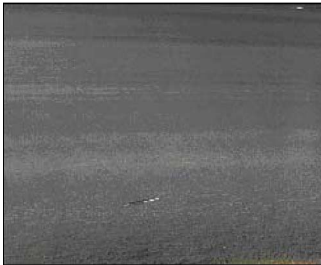
Figure 2.44: Example of segregation [Caltrans 03]
