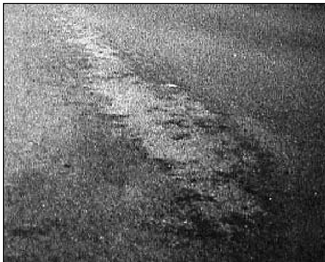
Figure 2.46: Raveling damage caused by premature exposure to traffic [Caltrans 03]
