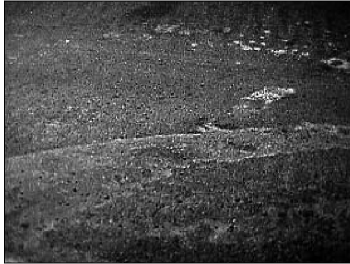
Figure 2.47: Damage resulting after heavy rain in a high traffic location [Caltrans 03]
