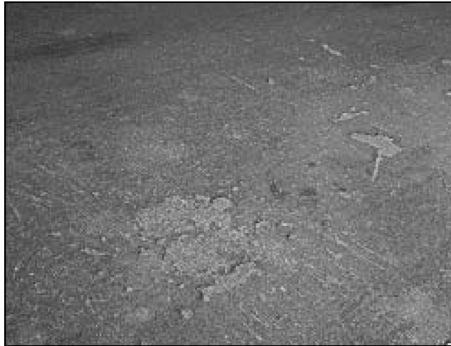
Figure 2.45: Example of delamination resulting from a False Slurry [Caltrans 03]
