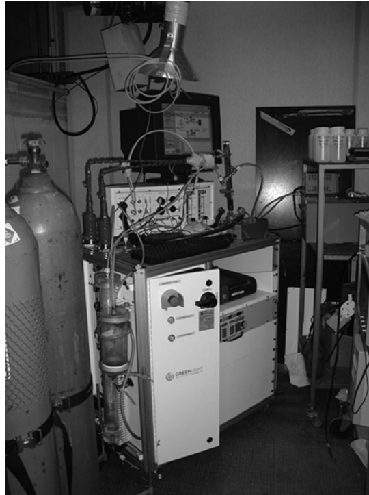
Figure 2-3: Greenlight Power Technologies, G-50 Fuel Cell Test Station
