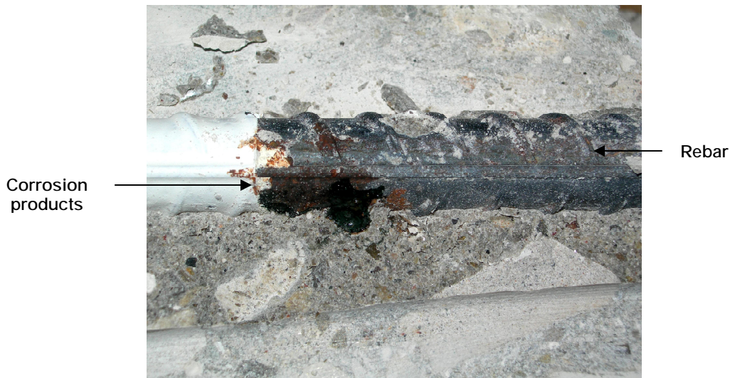
Figures 4-29, Steel rebar condition in R_1 concrete prism, 380 days after exposure.
