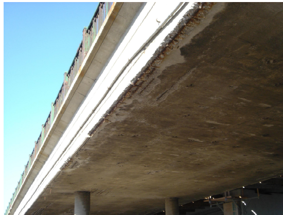
Figure 3-1, Deteriorated Townline Road bridge over highway 401 before demolition.
