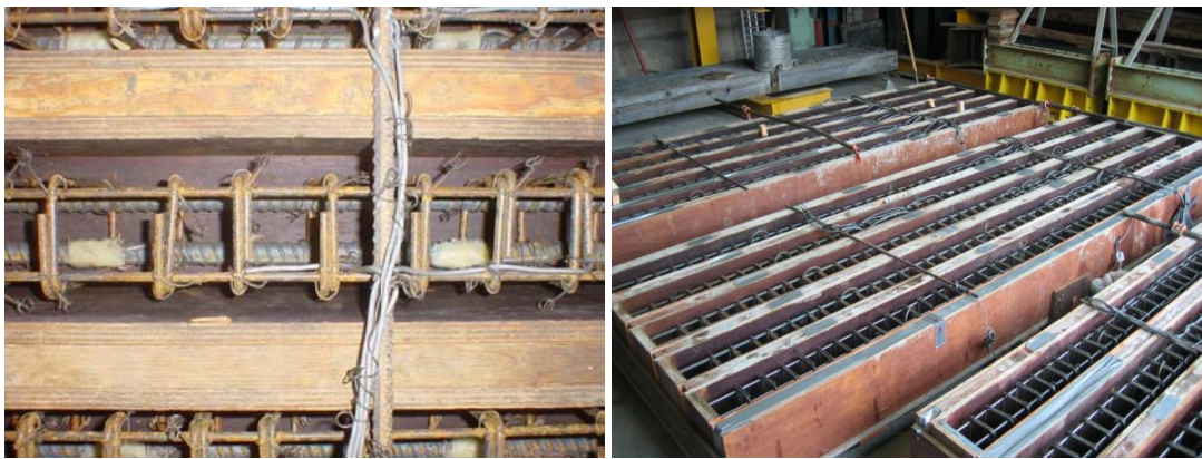
Figure 4.7: Strain gages covered with wax (left) and steel bars inside the timber forms (right)
