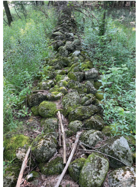
Figure 77: Image of a decaying loose stone wall as Third Order Nature , near Glenn Morris, Ontario. 2023, Photo by author.
