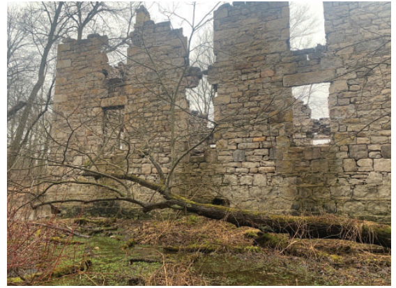
Figure 38: Image of The German Woolen Mill in a state of advanced decay near Paris, Ontario. 2023, Photo by author.
