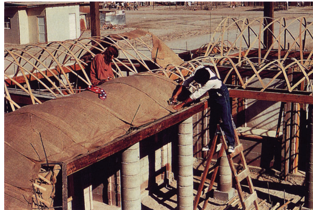
Fig. 1.2 In Mexicali, houses with lightweight vaulted roofs were constructed using woven baskets made of thin lattice strips with burlap and chicken wire stapled to them, and then plastered over.
