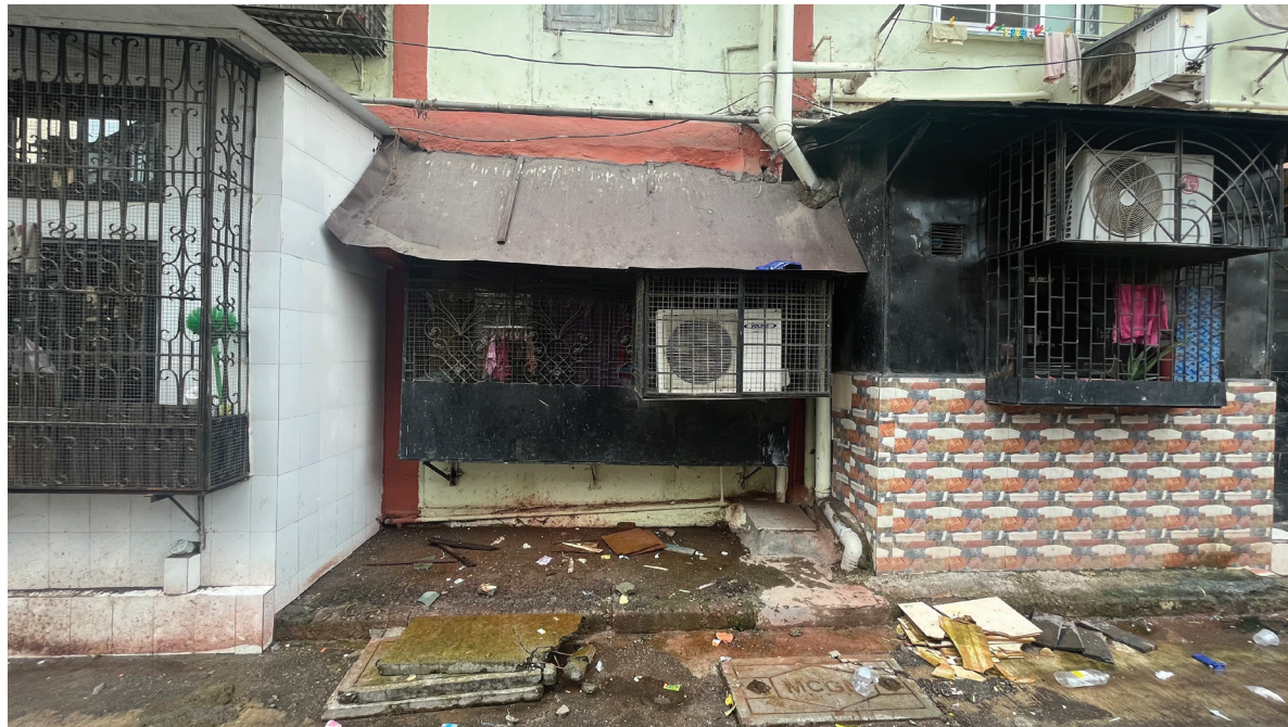
Fig. 4.41 The decay of facade BIT Chawls
