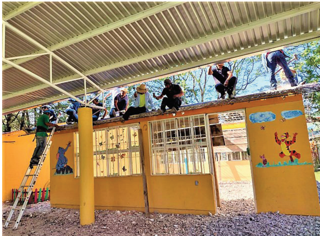
Fig. 1.1 Parents rebuilding a classroom in the San Juan Achiutla kindergarten damaged by the 2017 earthquake, Oaxaca, Mexico, 2021.
