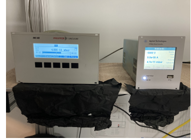
(c) Pump, pressure monitors.
