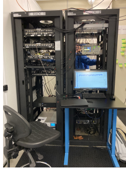
(b) Electrical racks.
