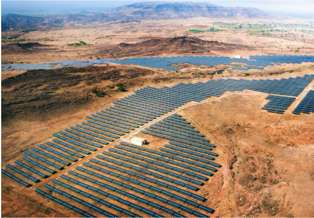
Figure 1.1: Badhla Solar Park - 2245 MW PV Plant in Rajasthan, India [23]
