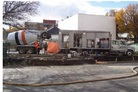
Wet Mix Equipment
