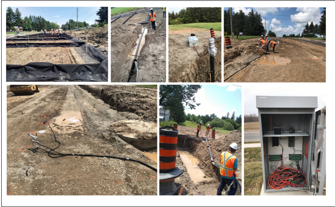
Figure 4.21: Notre Dame Drive cabling and data logging station
