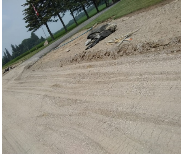
Figure 4.20: Settlement on granular A at LCC400 section
