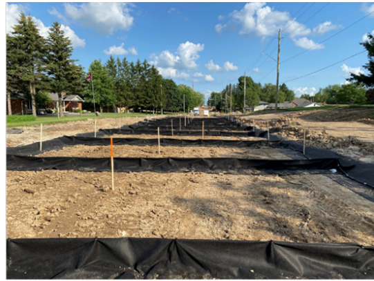
Installed Baffles for LCC
