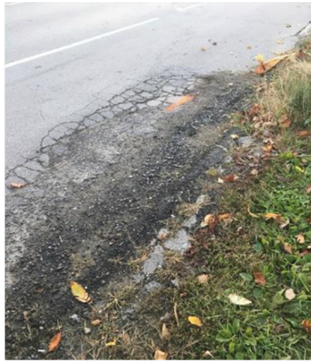
Pavement distress at bus stop (Erbsville)
