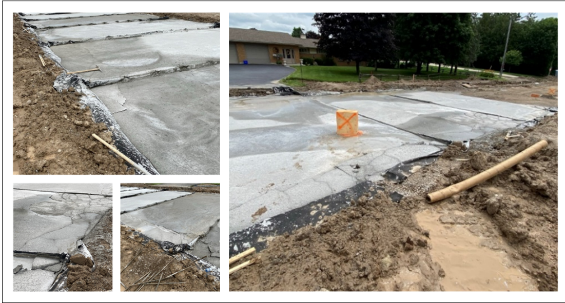
Figure 4.18: Water accumulation and cracking close to LCC400 sensor location
