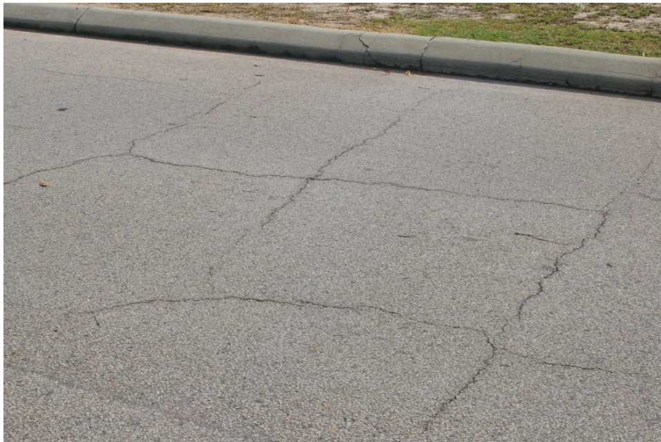
Figure 3-5: Block cracking in asphalt pavement
