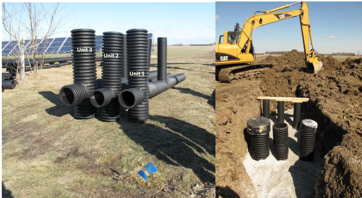
Figure 3.3. In-line monitoring units were installed to allow monitoring of the field tiles and surface drain.
