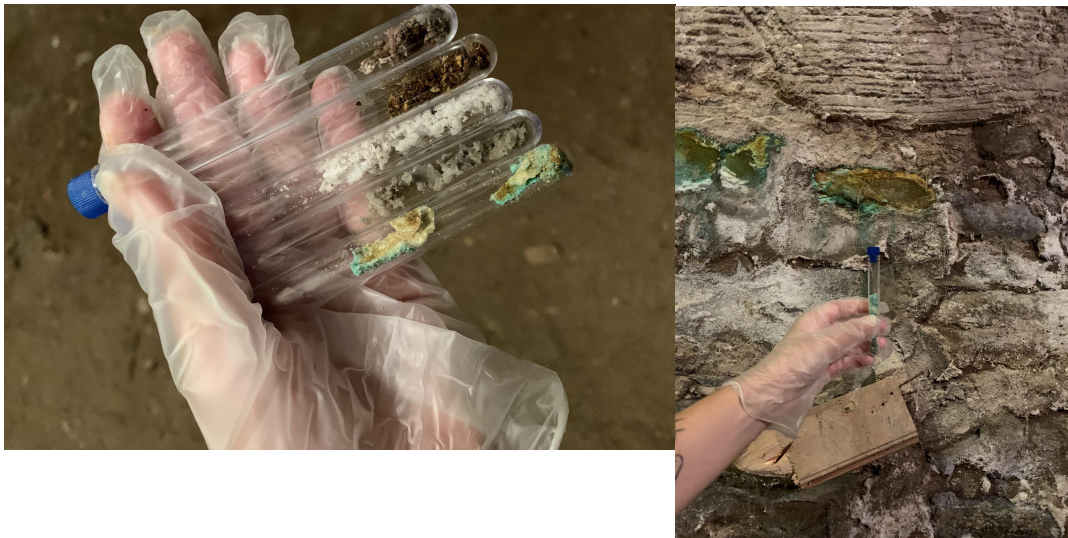
Fig 15. + 16. Maria Simmons, documentation of efflorescence samples, 2020.
