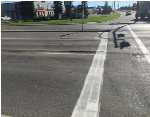
a. Pavement Rutting (Johnston et al., 2017)
