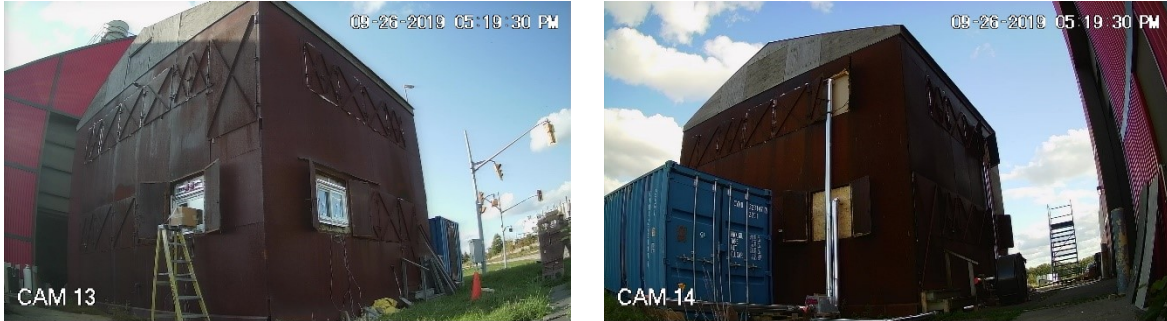
Figure 3.2: External view of the SE (left) and NW (right) corners of the UW burn house
