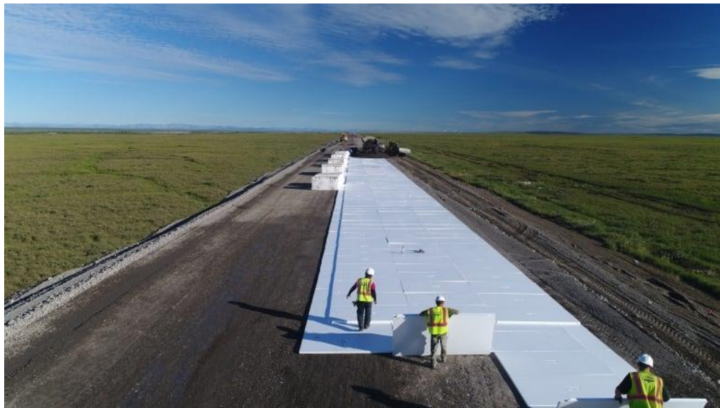
Figure 4.2. Polystyrene sheets being layered on the road subgrade during construction (M-Lepage et al. , 2012).
