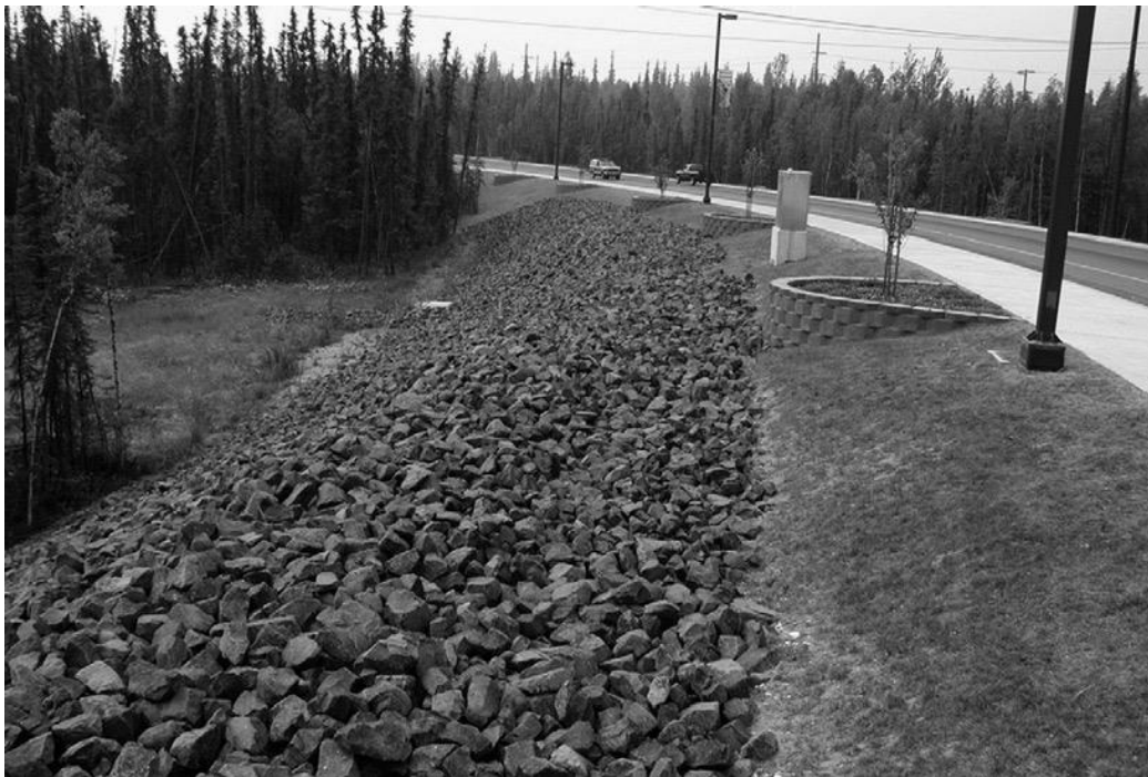
Figure 4.14. Air convection embankment installed along Thompson Drive in Fairbanks, Alaska (Xu & Goering, 2008).
