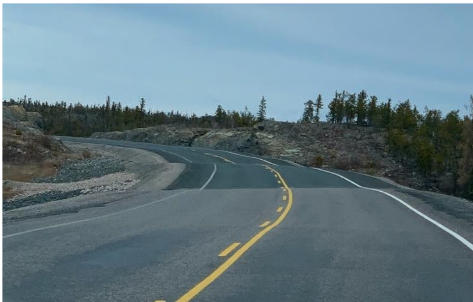
Figure 2.6. Differential settlement observed along the Ingraham Trail.
