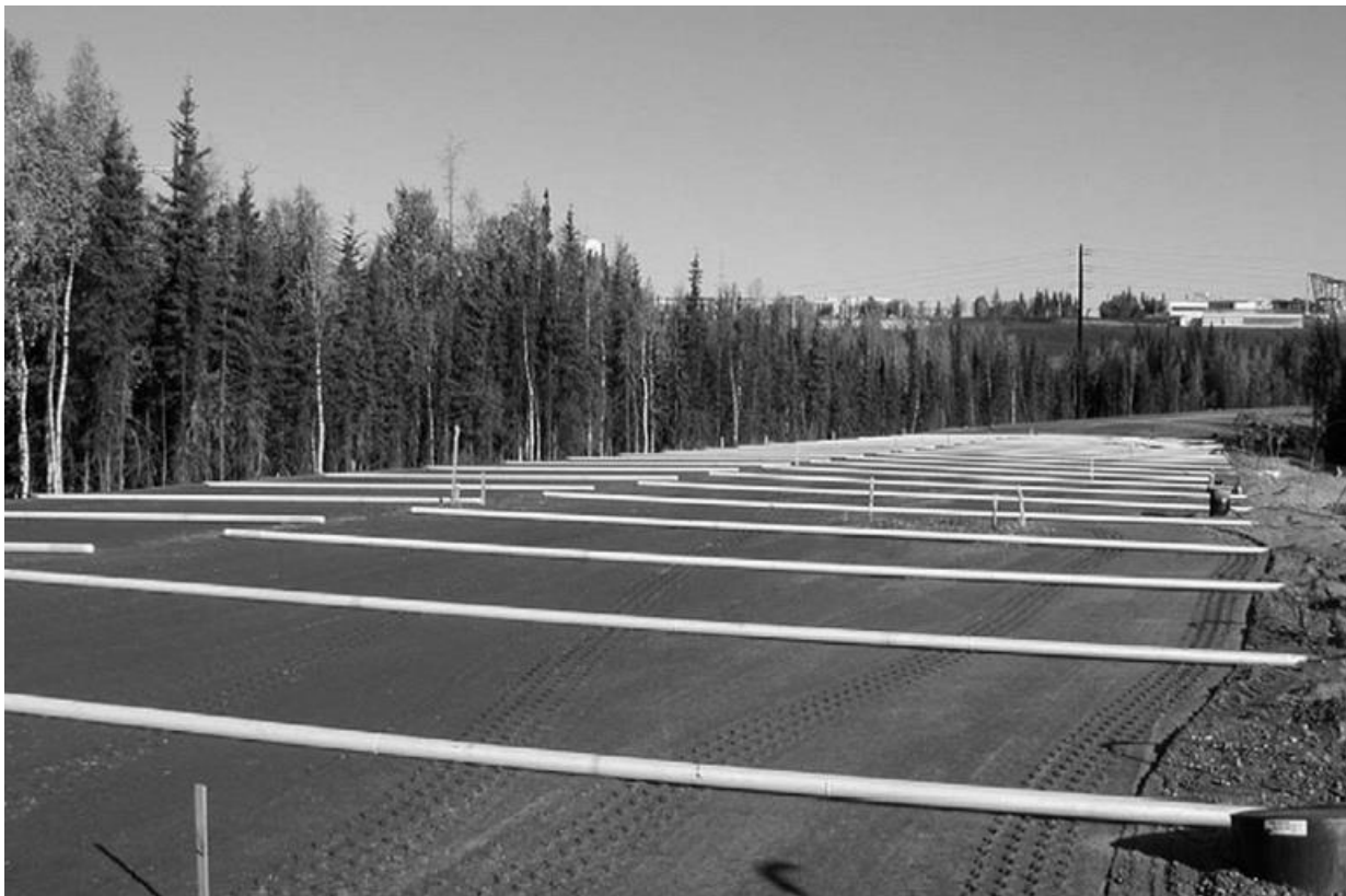
Figure 4.11. Hairpin thermosyphon condensers installed during Thompson Drive Construction (Xu & Goering, 2008).
