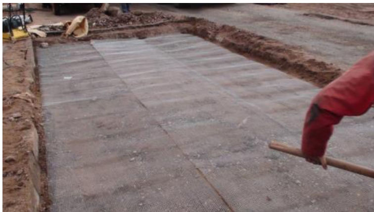
Figure 4.17. Geotextile being installed in the subgrade of QTH (Li, Zhi, Fang, & Zhang, 2013).
