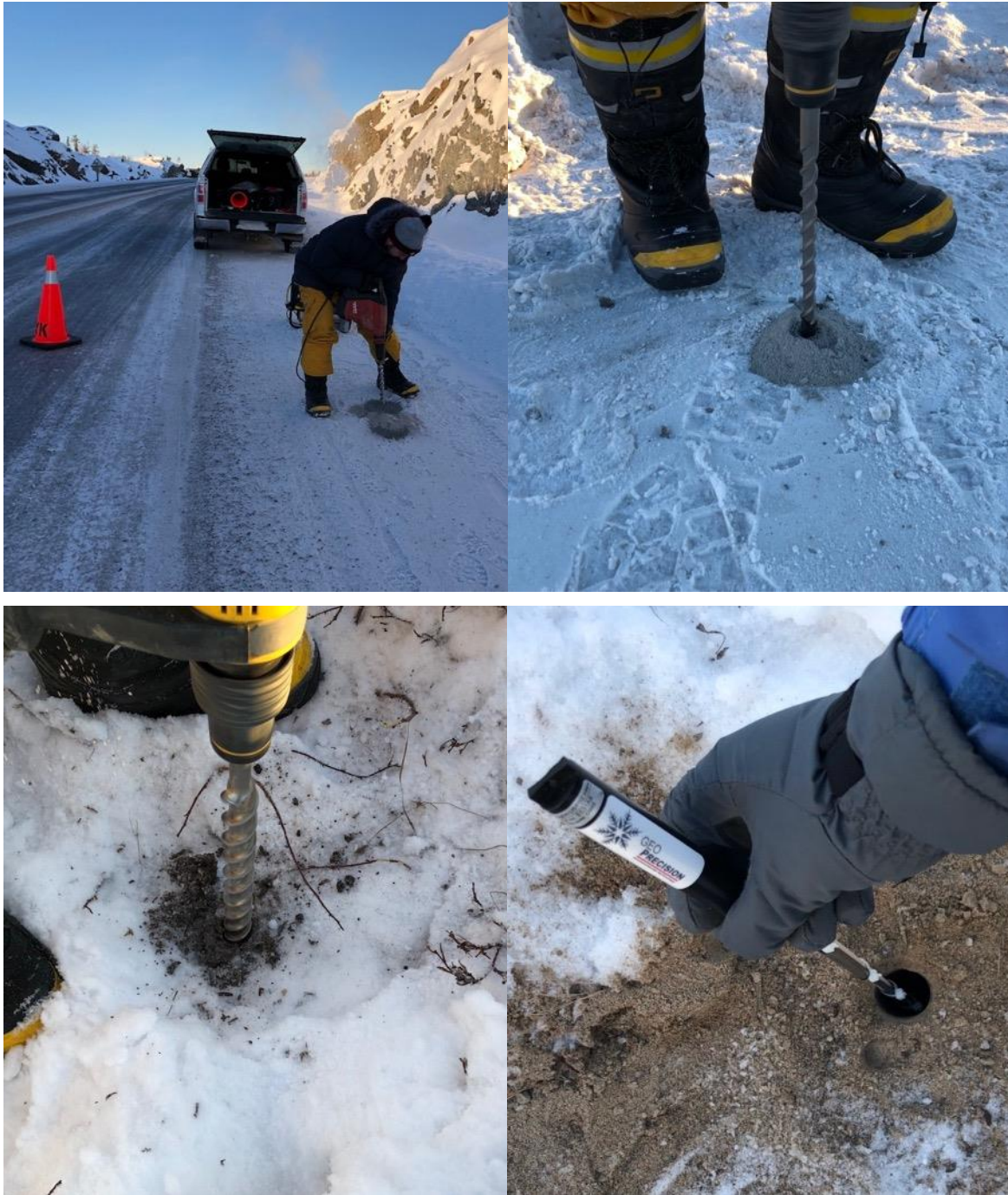
Figure 3.4. Drilling (top left, top right, and bottom left) during field installation and insertion of thermistor assembly (bottom right).
