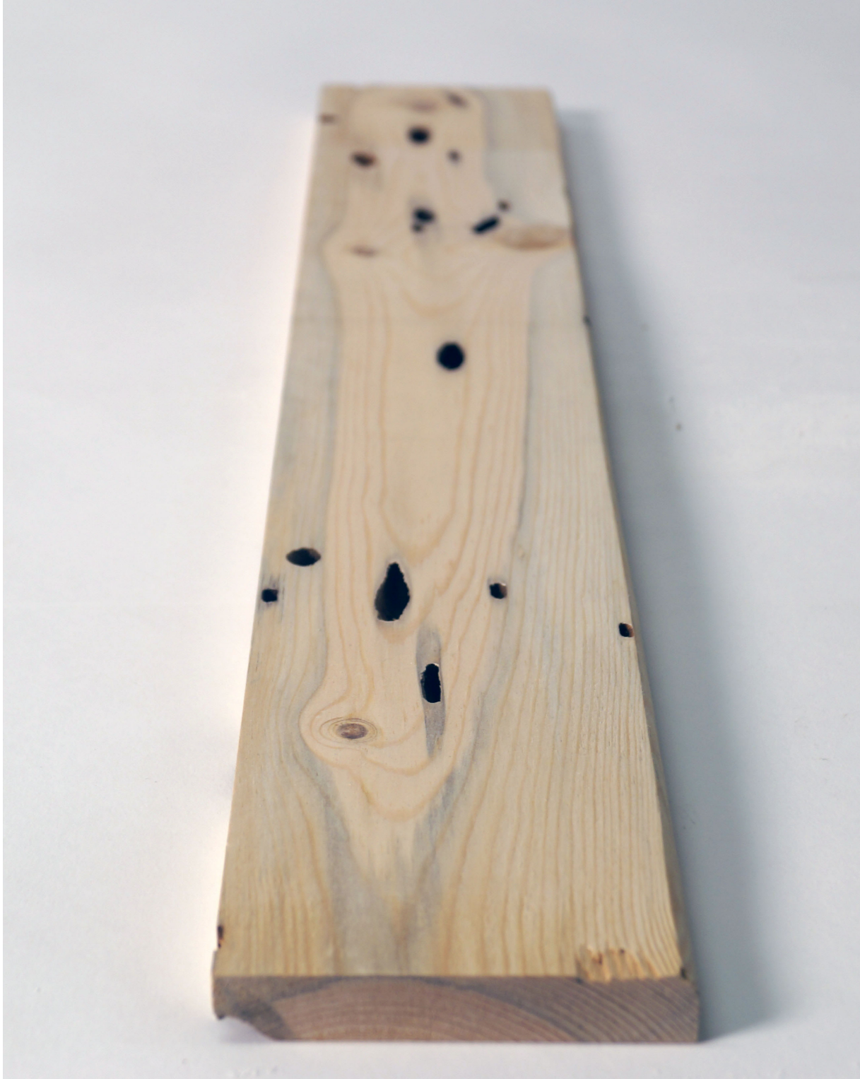
Figure 2.12 - Beetle infested SPF lumber - Found in a local building supply store among other dimensioned lumber by accident. This is certainly not the mountain pine beetle but a blue fungus is noticeable having accompanied the beetle that has eaten into this wood.
