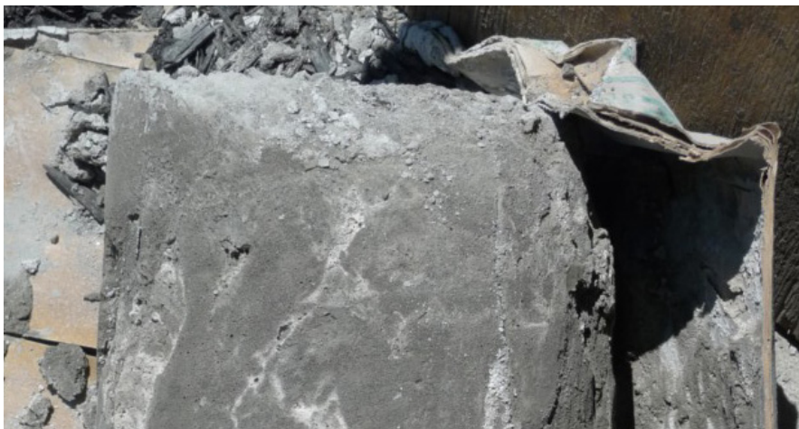
Figure 0.2 Top of low-density sanded foam concrete prepared in a batching plant. Significant segregation is evident.
