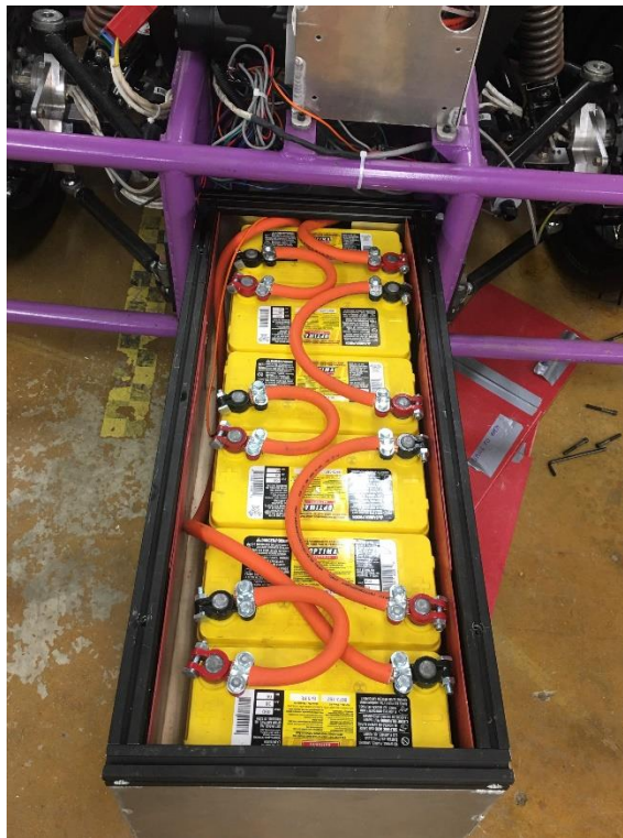
Figure 3.2 The Urban Vehicle's High Voltage Battery Pack
