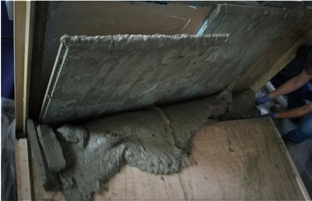
fig. 18 Formwork breaks open from lateral pressure of concrete revealing semi-hard mix and foam cavity
