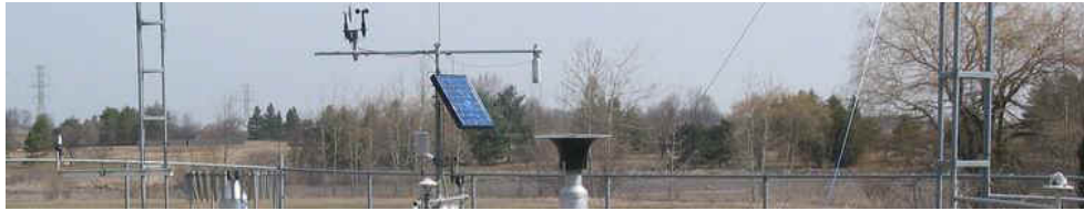
Figure 3.2: EC weather station located at the University of Waterloo. Image source: wwaterloo.ca
