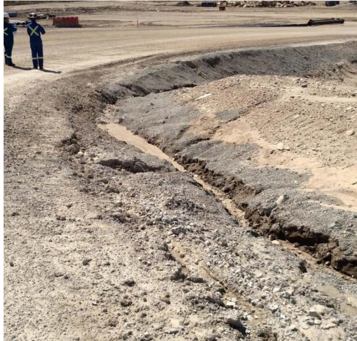
Figure 5 Localized Shoulder Washout
