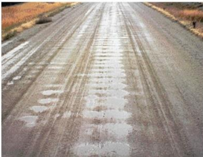
Figure 6 Centerline Wash Boarding on Gravel Road (Skorseth & Selim, 2005)
