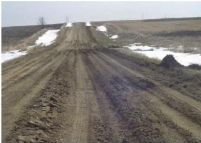
Figure 8 Severe Rutting (Zhang, 2009)
