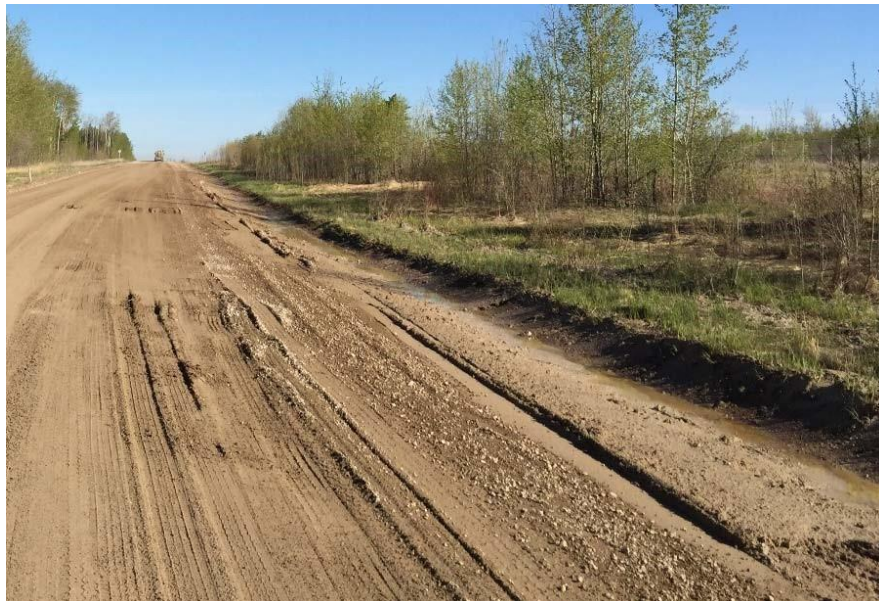
Figure 27 Washboarding and Soft Spots in Canterra Road
