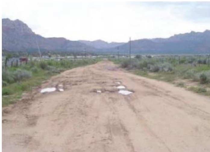
Figure 7 Potholes on Wheel Path (FHWA, 2015)
