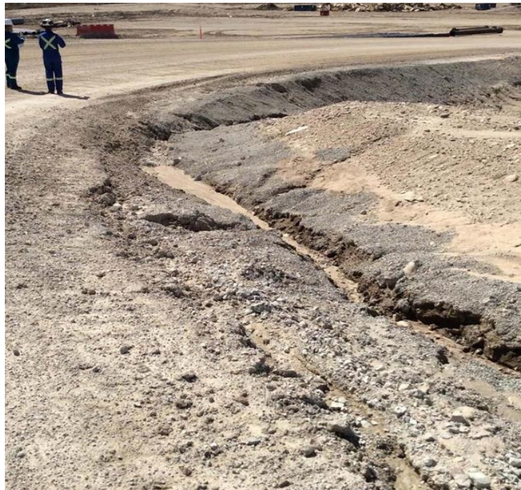
Figure 23 Local Washout on Pit Road 4 Section
