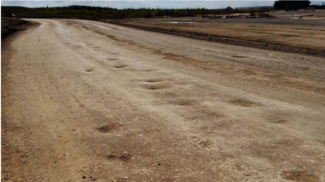
Figure 25 Distresses in OPP2 Access Road Section (Washboarding and Potholes)
