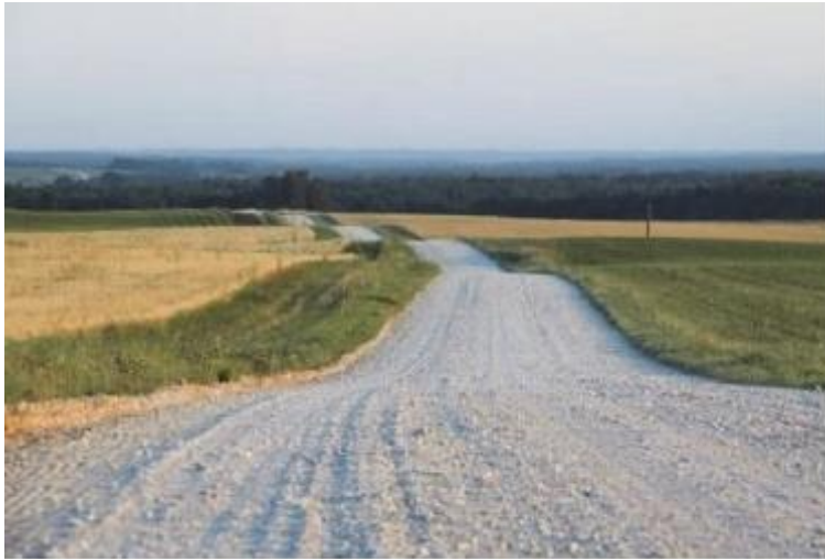
Figure 3 Loose Aggregate on Roadway (Zhang, 2009)
